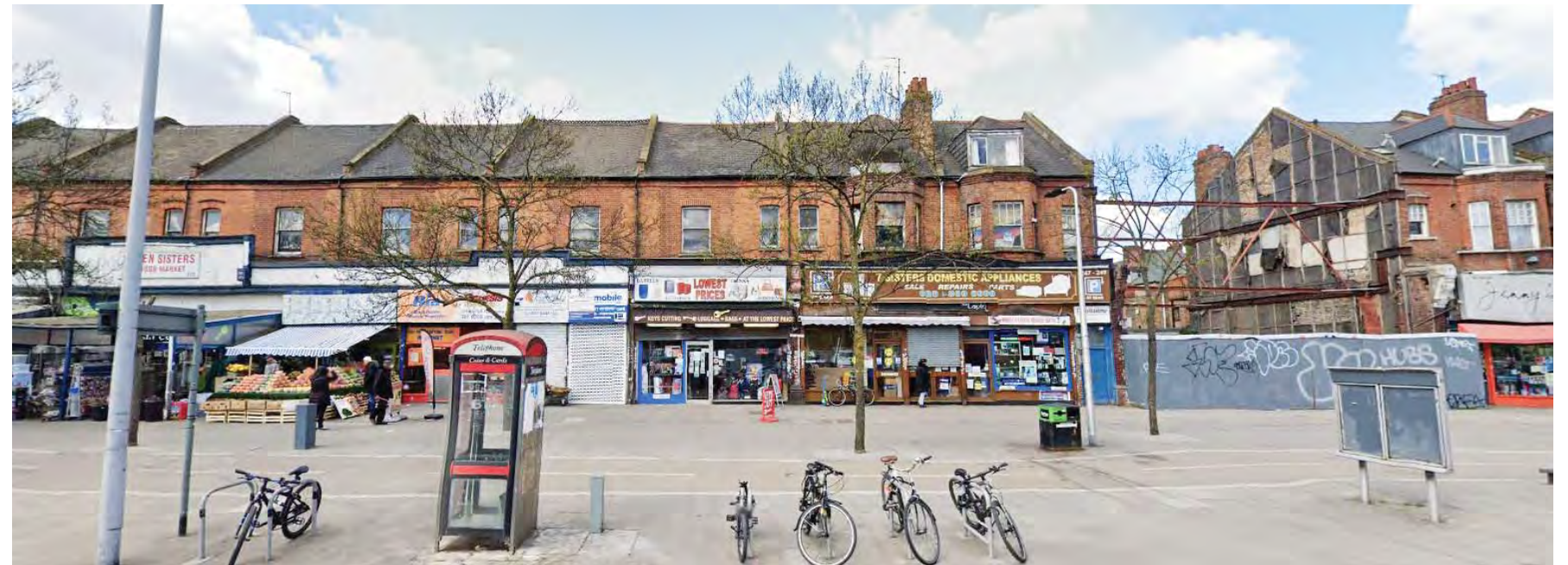
7. View of 245 - 247 - 249 High Road with the demolished adjacent plot with temporary truss' spanning between party walls.
