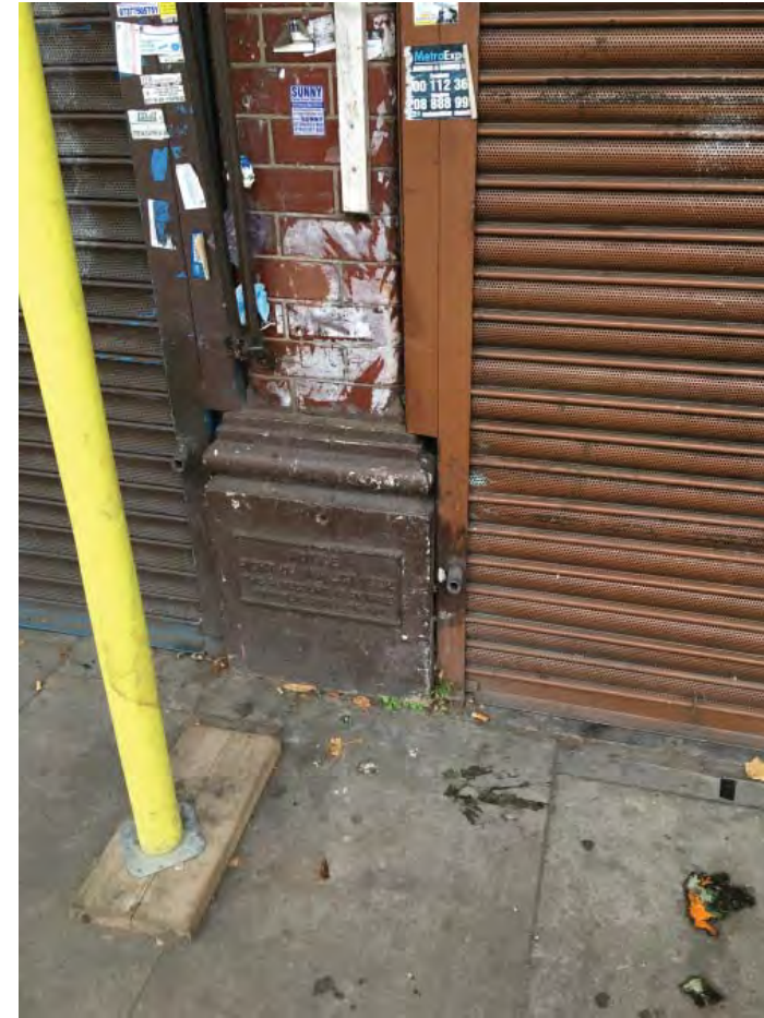
15. Existing junction of roller shutter guide and glazed tile pillar plinth of no. 245 High Road.
