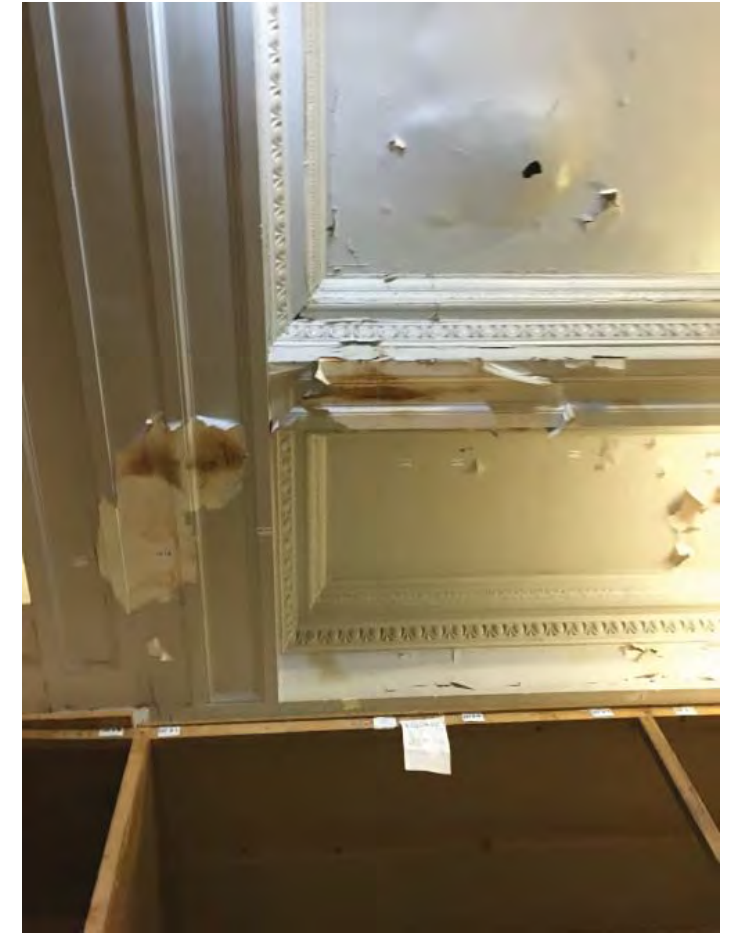
16. Water damage to ceiling of 245 High Road due to life expired waterproofing.
