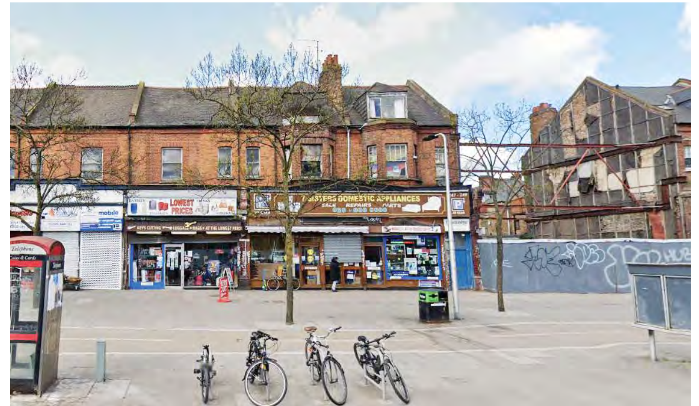
1. View of existing elevations of 245, 247 & 249, 249a and adjacent vacant plots of 251 & 253 with temporary propping.
